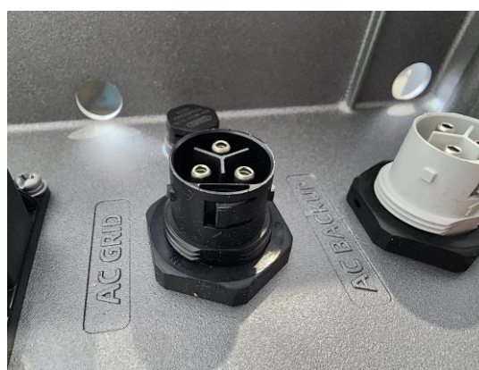
AC port view with block cover removed
